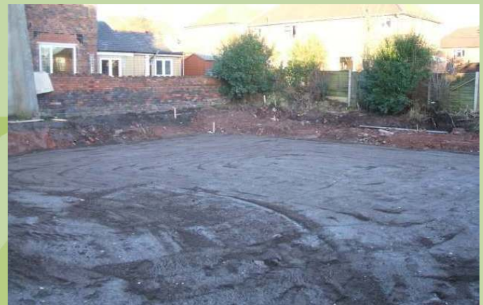
With the Geotextile Membrane in place and covered, work is able to continue unhindered.
